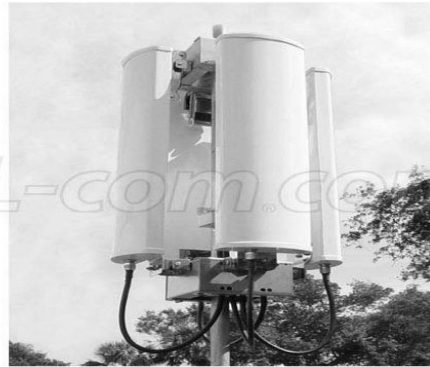
Figure 1: Four Panel antennas mounted on a tower.
