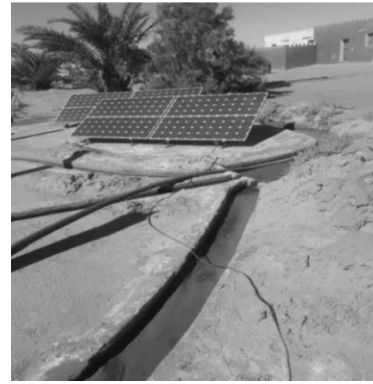
Figure 16. Photovoltaic pumping in the Amguid-Tamentit site [48]
