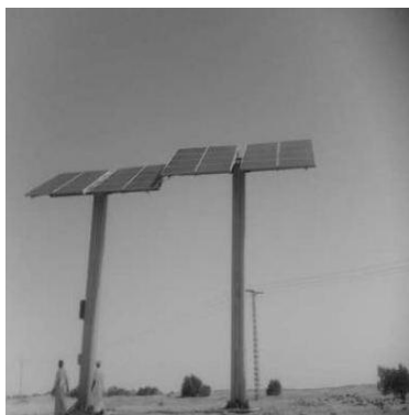
Figure 15. Photovoltaic pumping in the Ait Messaoud site [48]
