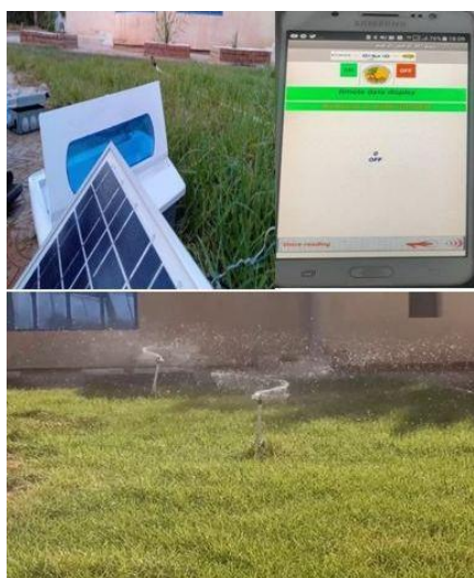
Figure 11. Agricultural smart irrigation system, using the application of remote control
