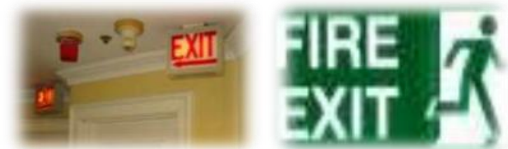
Figure 7. Various guiding signs directing building users in the corridors to the escape exit [9]
