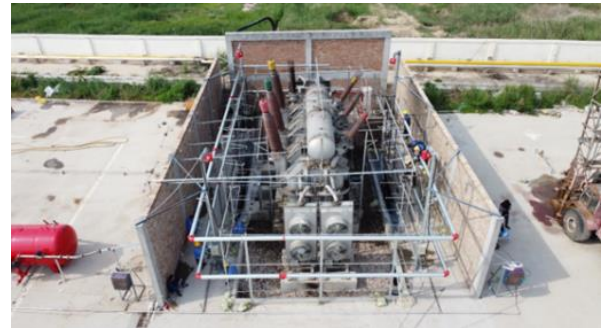
(a) \pm 220 kV oil-immersed transformers
