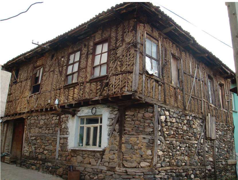
Figure 15: Turkish traditional house with the ground floor made of stone with some wood insertions, and the upper floor made exploiting the humuş system.
