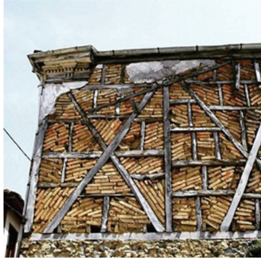
Figure 16: Detail of an upper floor humuş with brick filling between timber frames.
