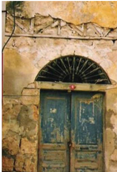
Figure 17: Fallen lime plaster put in sight the humuş system of the upper floor.
