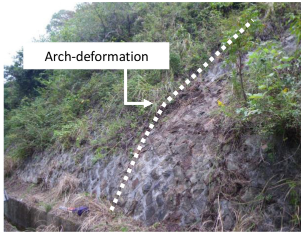
Figure 1: Example of an arch-deformed masonry retaining wall.
