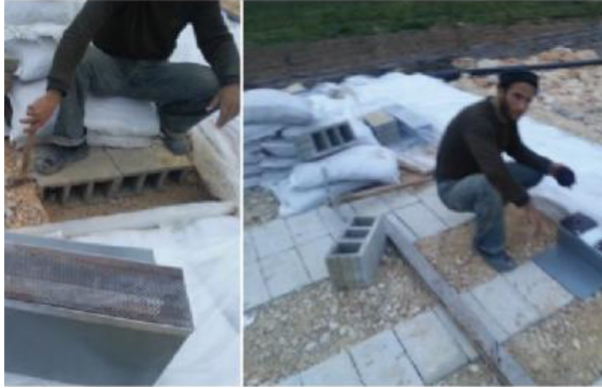
Figure 5: Earth duct outlets.
