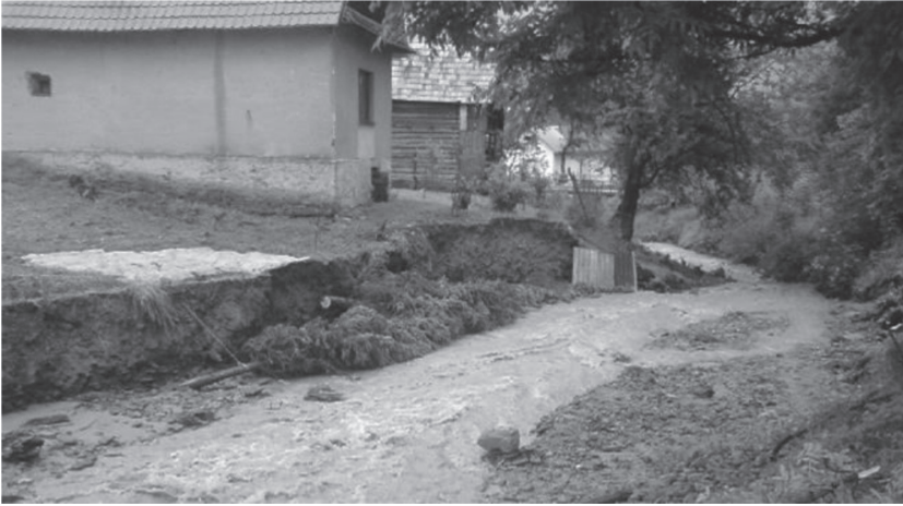
Figure 2: Alternative 0 (A0): stream bed will not be regulated – the current state (photo: June 2010, flood).
