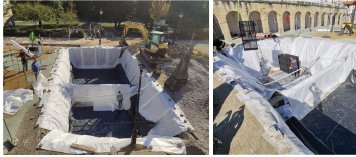
Figure 6: Details of the stormwater tank (image by Marc Rips).
