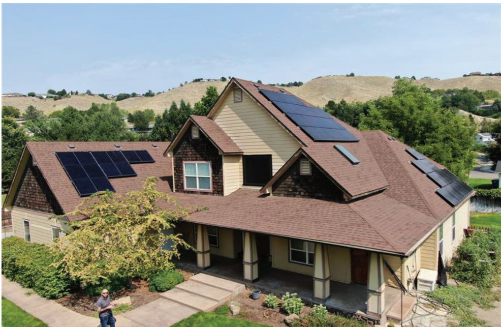
Figure 3: Completed solar system installation on the rooftop of a Boise area home. Photo courtesy of Blue Raven Solar Systems, Salt Lake City, Utah.
