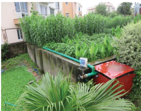
Figure 7: Satya Sai Sikshya Sadan school – the well-functioning constructed wetland, September 2019.
