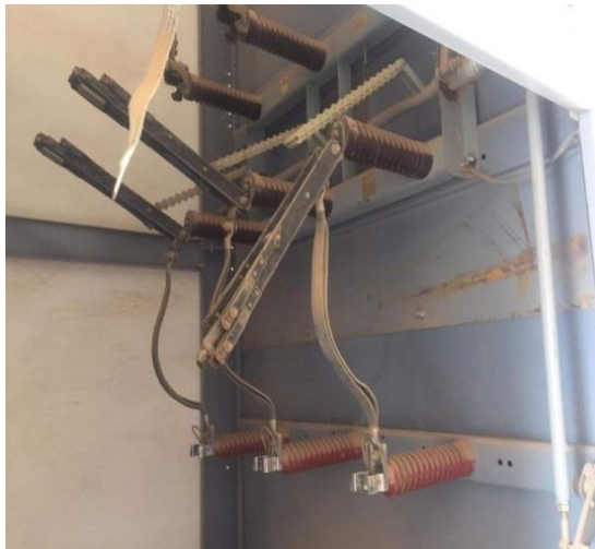
Figure 2. Classic protection cell switch
