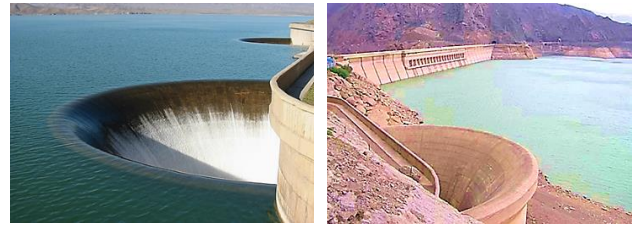
Figure 1. An example of a sectoral morning glory spillway constructed in the Manjil dam (Sefid Rud River Dam) in Iran [10-11]
