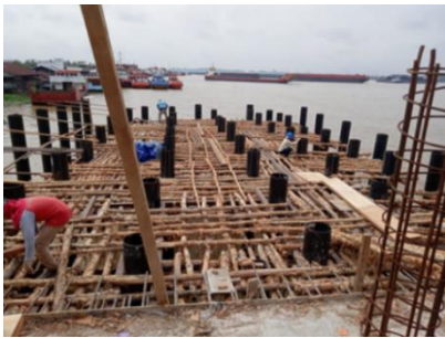
Figure 1. The use of galam wood as formwork which is not arranged systematically
