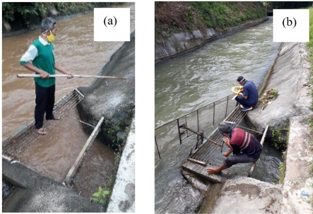
Figure 10. (a) Existing vertical trash rack (TV-E), (b) Horizontal Trash rack Diverter Trash (HTDT)
