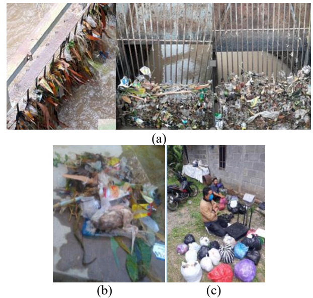
Figure 6. (a) Solid trash clogging at the vertical trashrack (b). Solid trash at the intake mouth, solid trash at the watergate before the turbine basin, (c) Weighing the intake clog and turbine trash (1-30 June 2020)
