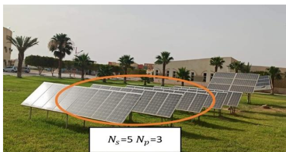
Figure 3. The photovoltaic field
