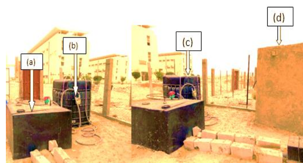
Figure 1. Biodigester constructed at the Faculty of Science and Technology (FST): (a): digester, (b): flowmeter, (c): gasometer and (d): shelter for testing
