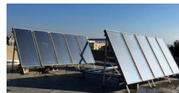
Figure 1. Flat plate solar collectors' arrangement
