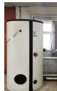
Figure 2. Water storage tank
