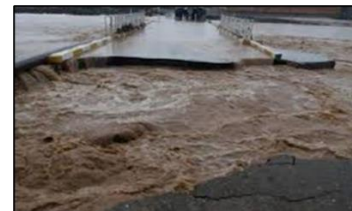
Figure 1. The collapse in Mousil Bridge North of Iraq
