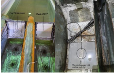
Figure 4. Strain gauge on gate and dam body dam
