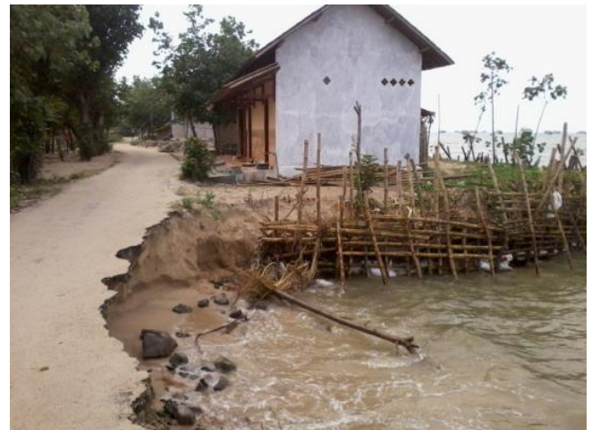
Figure 9. Road damage in Kragan village due to abrasion
