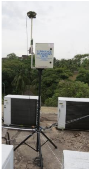
Figure 5. The external illuminance sensor is located on the building's roof
