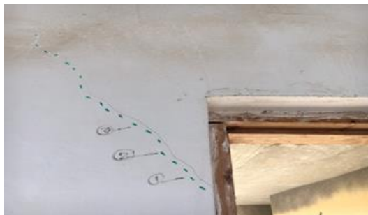
(a) Crack near door No.1
