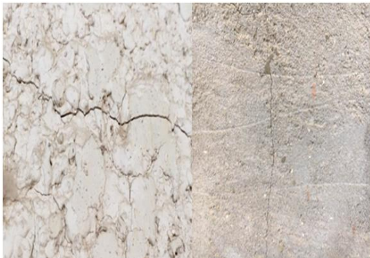
Figure 12. Building BX - cracks recording and monitoring on walls
