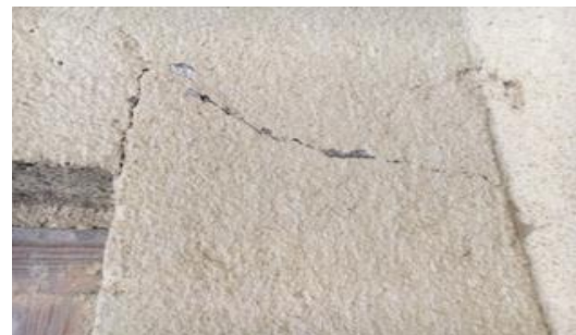
(b) Crack near door No.2
