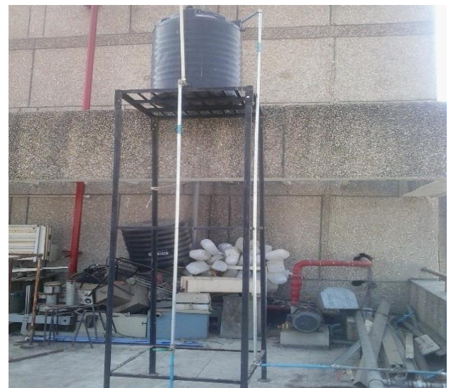
Figure 1. Hard water tank
