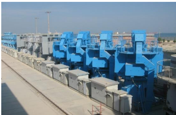
Figure 1. Part of the pumping station under study
