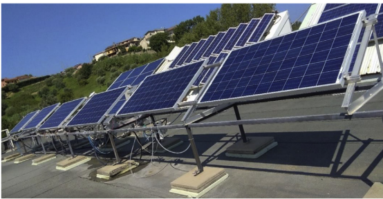
Figure 2. Experimental apparatus on the roof of a building of the DIMEG department at Unical [6]
