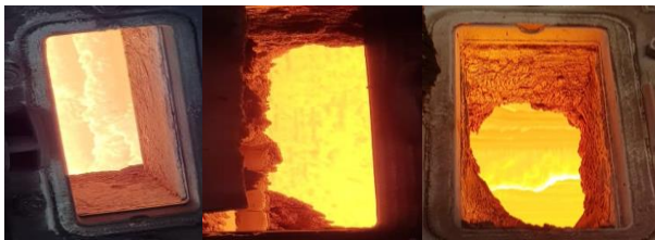
Figure 8. Coal ash inspection at boiler pendant tube
