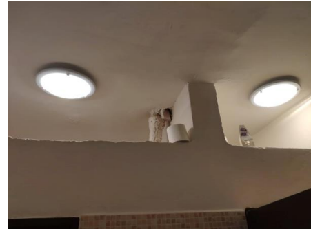
Figure 7. Former inefficient illumination design in sanitary area
