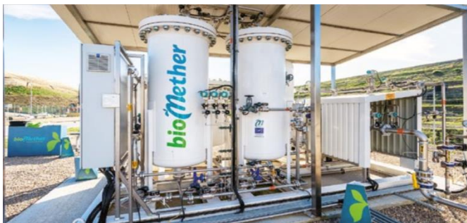
Figure 1. BioMethER pilot plant
