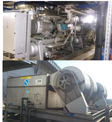
Figure 2. Machine room and cooling towers
