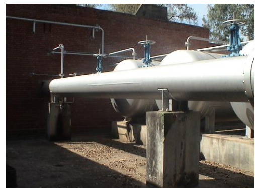
Figure 6. A picture of the storage tank
