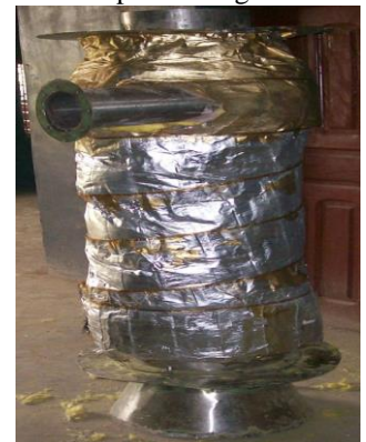
Plate 6: Lagged recuperator assembly
