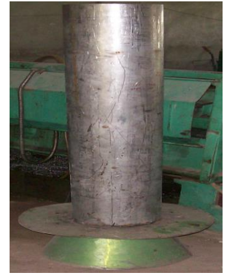
Plate 2: Recuperator inner radiant tube
