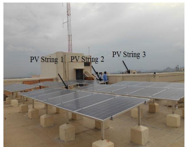
Figure 10. Solar panels installed in rooftop
