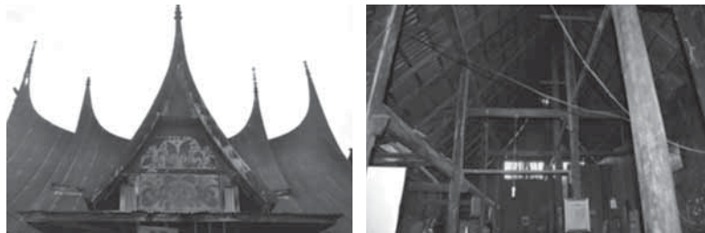
Figure 13: The curved roof provides ventilation and facilitate the flow of rain water.
