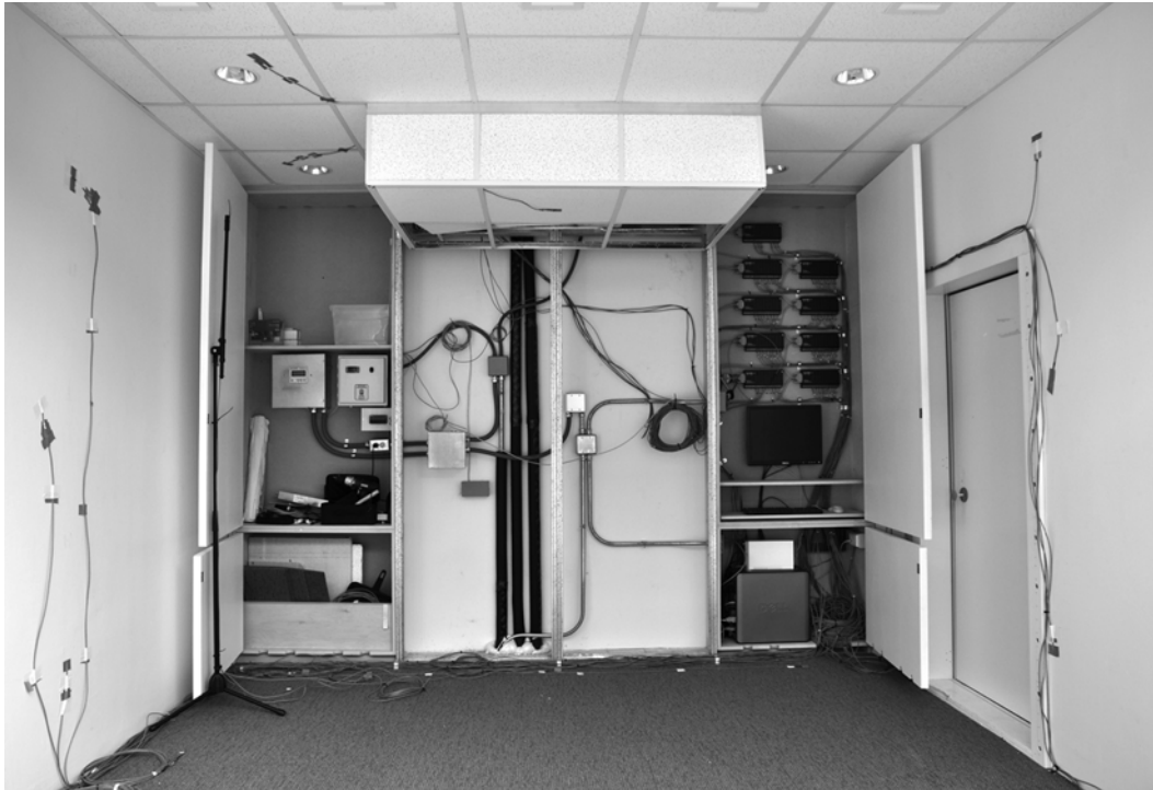
Figure 2: View of Facade Laboratory interior with remote sensor equipment.
