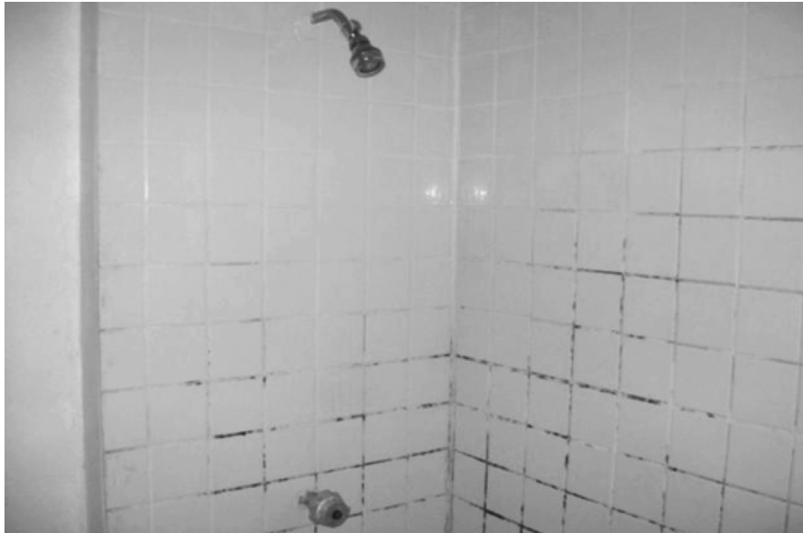
Figure 3: Shower tile with grout mildew stains.
