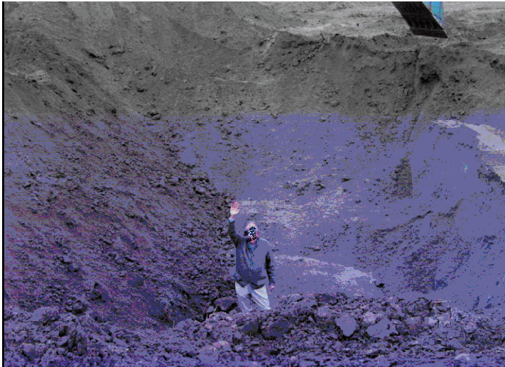
Figure 2: A large excavation in terrain supposed to be worked on for agricultural improvements.
