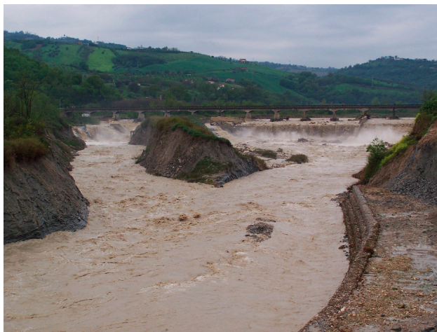
Figure 1: Erosion in a river in the Centre of Italy. Downstream from the bridge a checkdam has been built to prevent the bridge's collapse. However, over the years, the checkdam itself has had several problems. The origin of the erosion is believed to be excessive mining.
