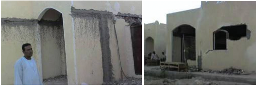
Figure 22: Cracks immediately appeared in some of the new houses in New Al Taref project. Source: www.youtube.com .
