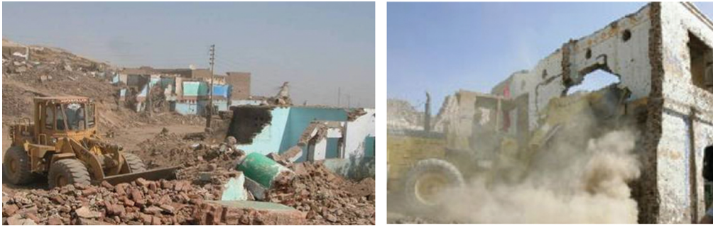
Figure 17: Destruction of Old Gournah in 2006 to force its residents to leave to the New Al Taref Village (the second version of New Gournah). Source: [10] and www.alarab.co.uk .
