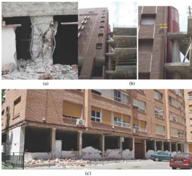
Figure 5: Damage from (a) short columns, (b) pounding and (c) soft floors. Source: Authors; Cartagena Fire Department.
