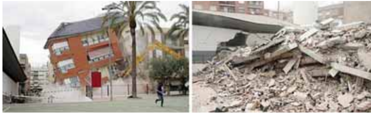
Figure 17: Unexpected collapse of the building (left) and fall onto the nearby church (right). Source: RTVE.
