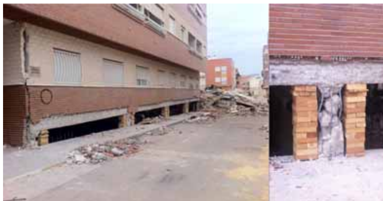
Figure 14: Situation of a building next to the collapsed one (left) and status of its short columns (right). Source: Authors.
