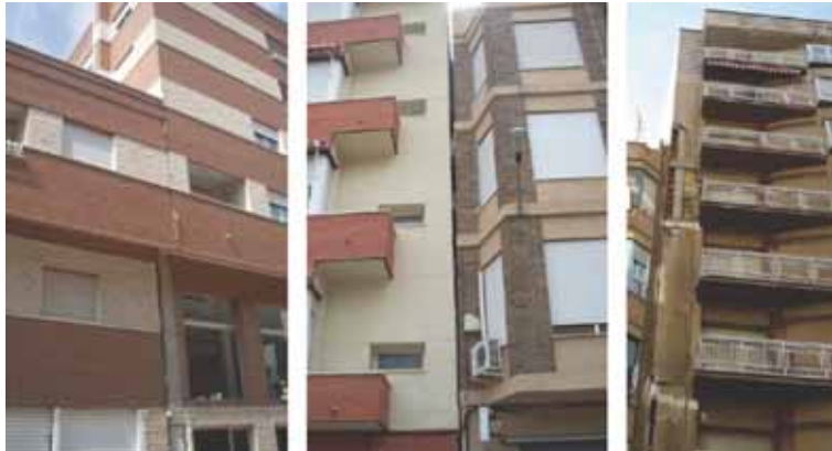
Figure 15: Different cases of buildings in Lorca with pounding and interaction between buildings due to height difference. Source: Authors.
