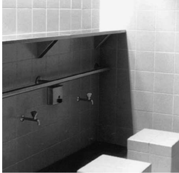
Figure 1: Example of an ablation station (terminal one, Dubai Airport).
