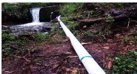
Figure 3. 100mm PVC penstock pipe with forebay inset
