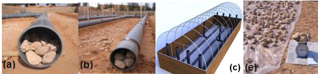
Figure 8. (a) and (b) Filling the pipelines with rocks, (c) Greenhouse structure and heating system, (e) Used rocks
