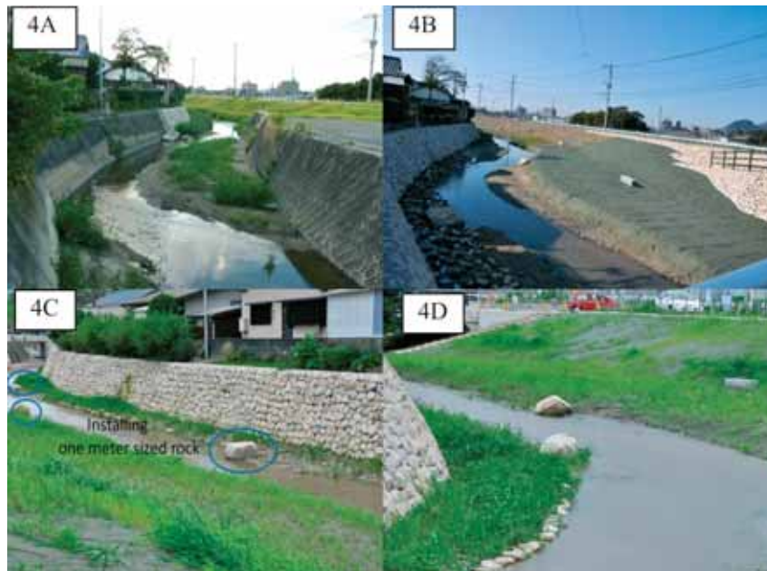
Figure 8: Station 4 condition. (A) Before restoration: the banks were lined by concrete. (B) Two months after restoration: revetments removed and river width doubled. (C) Installation of 1-m boulders. (D) Moderate bank slope.
