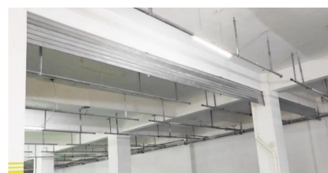
(a) Smoke retaining screen
