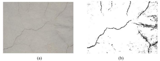
Figure 3. Image segmentation effects on different types of cracks
