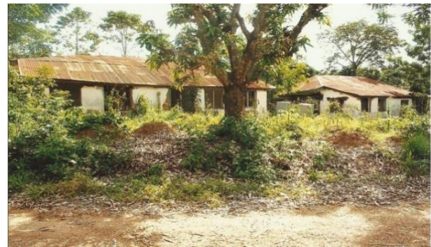
Figure 5. Abandoned buildings in the vicinity of the mine area occasioned by tremendous cracks due to vibrations resulting from mining operation
