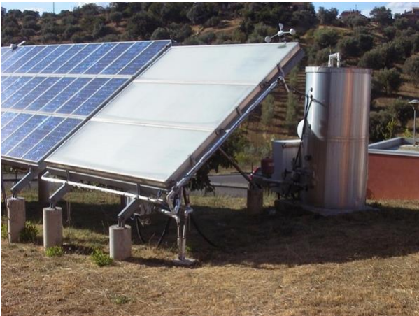
Figure 2. Thermal solar plant
