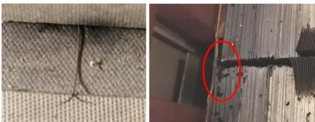
Figure 9. The photos on voltage regulating coil and core pieces
