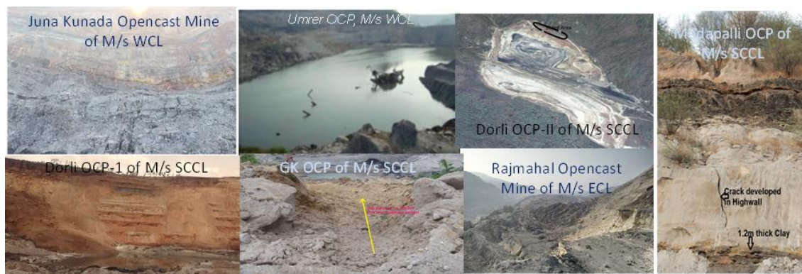
Figure 2. Photographs showing some of the pit slope failures in India
