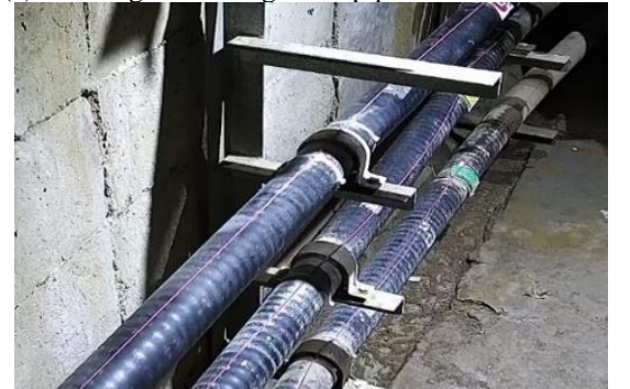
(b) An image of underground pipeline with defect
