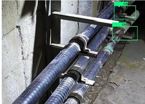
Figure 5. Recognition result of underground pipeline with defect
