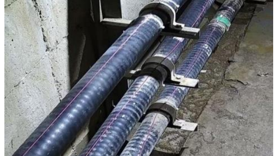
(a) An image of underground pipeline without defect
